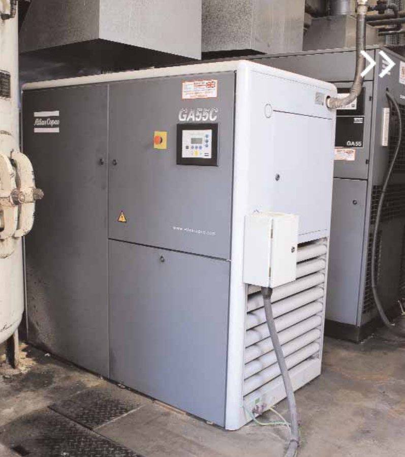
Typical large compressor house with multiple compressors
